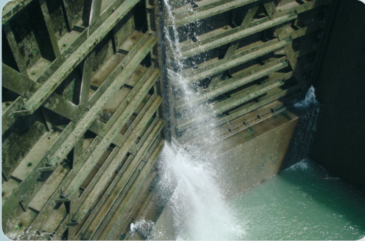
Beauchastel lock gate, 12 metres high (Rhône)
